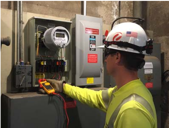
Xcel Energy technician installing the "net meter," a meter which measures when we sell excess power to Xcel Energy.
